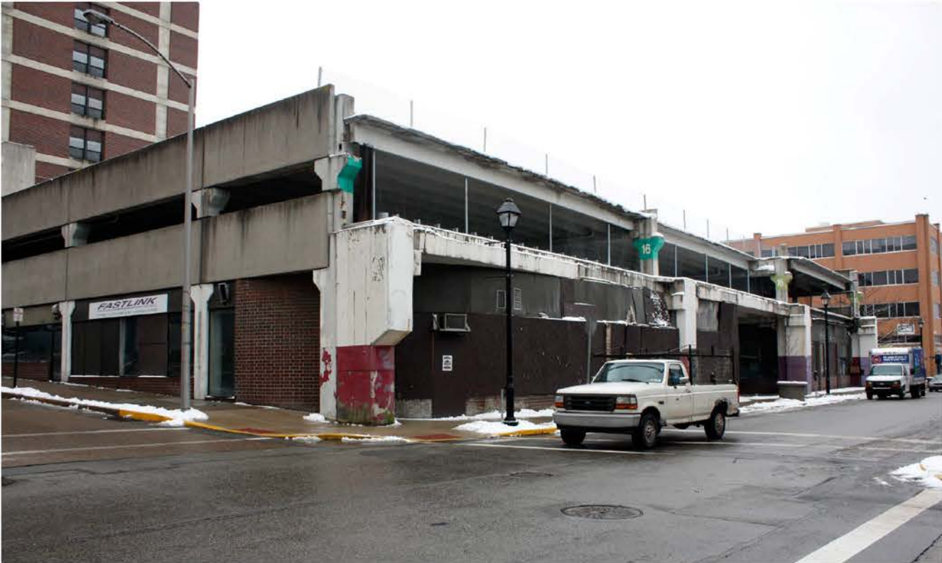
Figure 13 EXISTING BLIGHTED PARKING GARAGE ON 5 TH AVENUE
