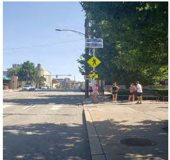
RRFB in front of Washington Elementary School – Allegheny County State Route 19
