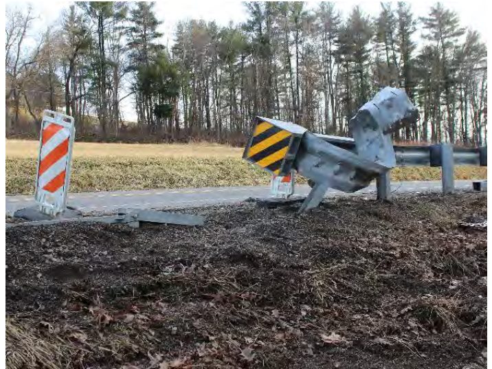
Guardrail damage on Route 28
