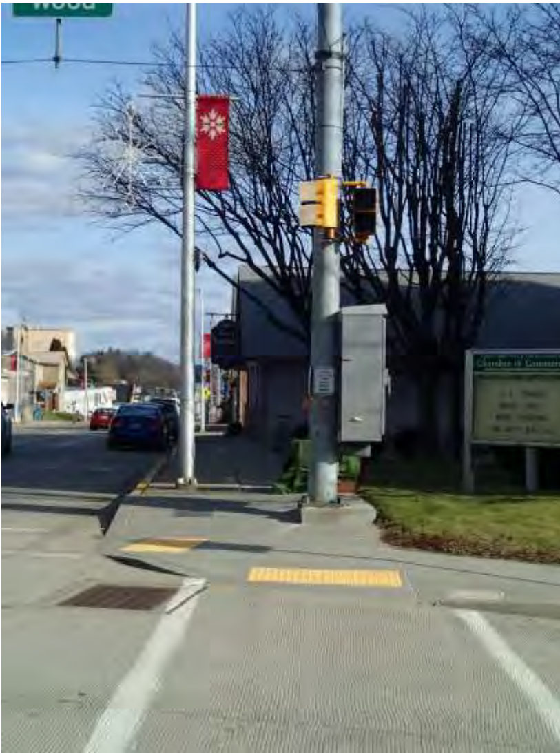
Sidewalks and DWS Present, Pedestrian Head Burnt Out
