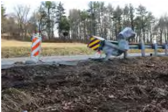
Used impact attenuator on southbound side of SR 28
