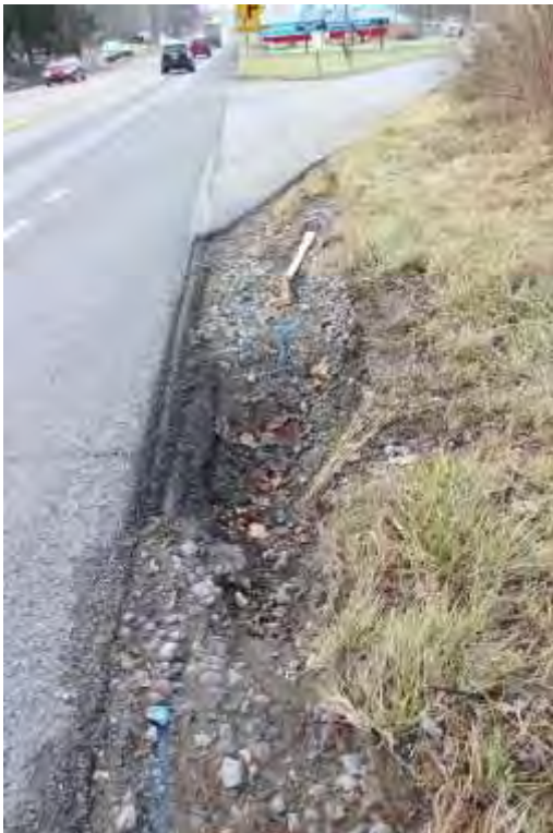
Roadside deterioration at McGregor Road
