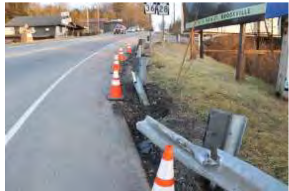
Damaged guide rail on SR 322/SR 28
