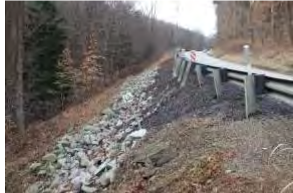
Damaged guide rail and slope repair
