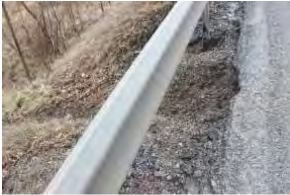
Heavy erosion on Section 742 of Route 28 from edge of pavement down to stream
