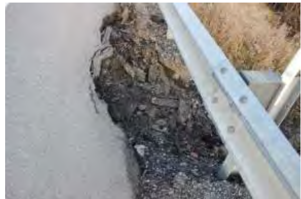
Heavy erosion under guide rail on northbound channelized right turn
