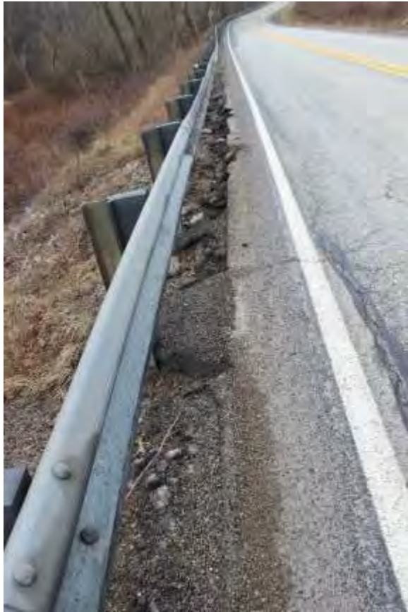
Erosion and deteriorating shoulder on northbound lanes of SR 28 (looking south)
