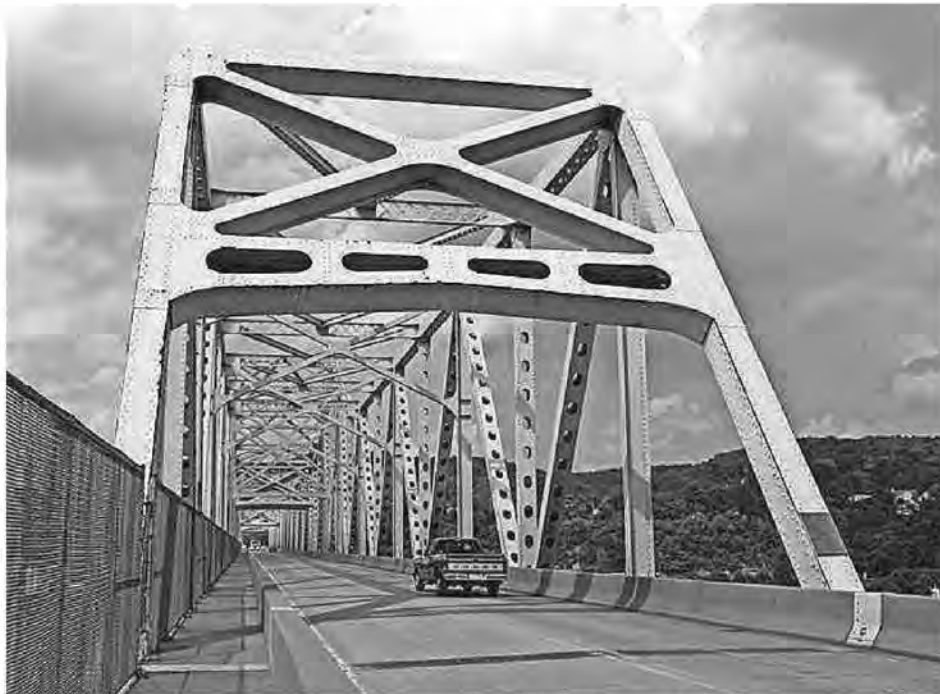
TIP will fund multiple projects, including fixing bridges in the region, including the Rochester-Monaca Bridge in Beaver County. HISTORICBRIDGES.ORG
